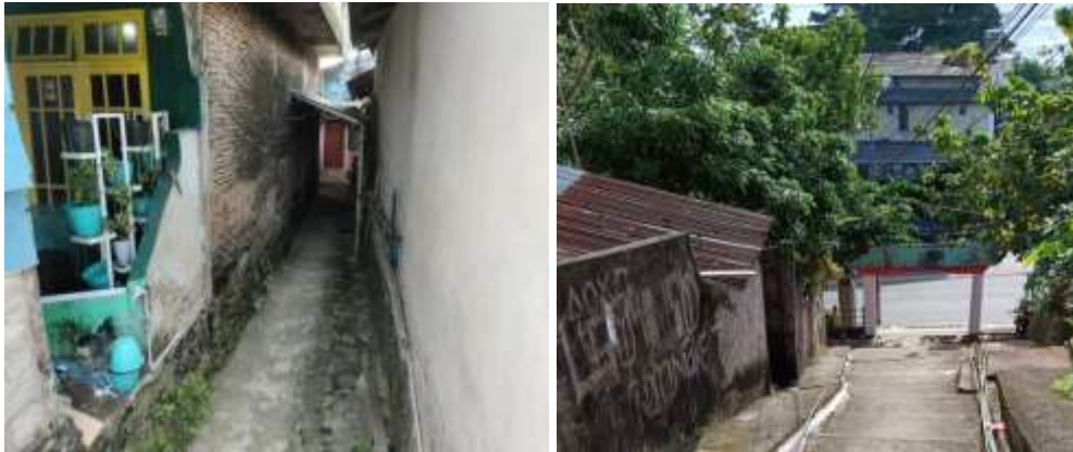
Figure 2. Condition of residential entrance roads Source: Observation Results, 2023
